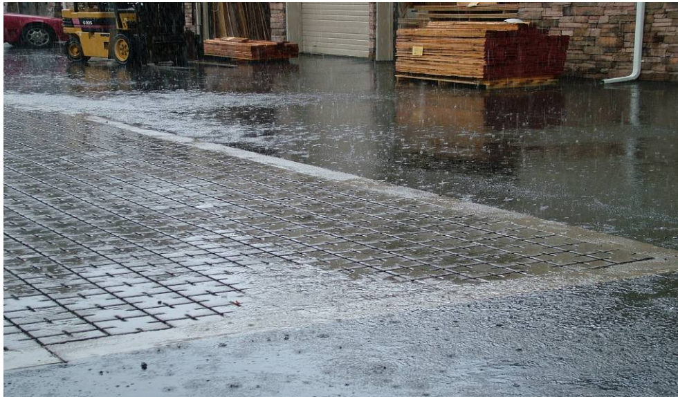
Figure 6. Water Running onto a VS 5™ Drain Permeable Pavement
